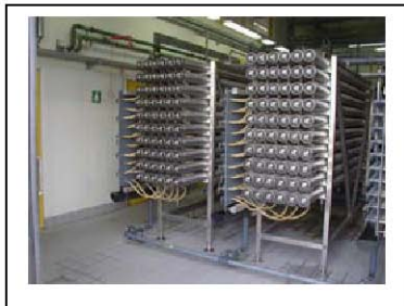
Reverse Osmosis Plant with Ultra Filtration Pre-Treatment
